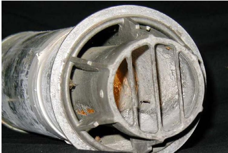
Figure 1: Example of corrosion in horizontal balanced flue
