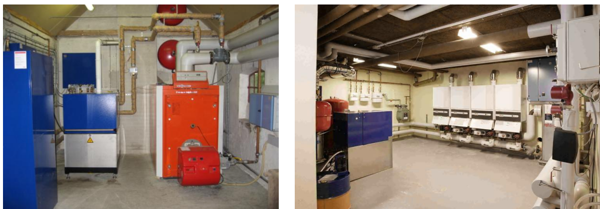
Figure 2 Two examples of a mini CHP unit system (EC-Power) installed in boiler houses
