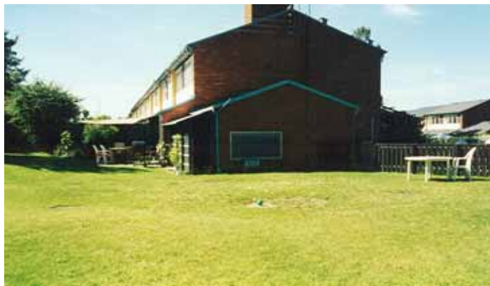
Figure 16 Two underground heat storage tanks are located below this lawn. A few covers can be seen in the grass. The cogen unit connected is placed in the lower building annex to the house end.
