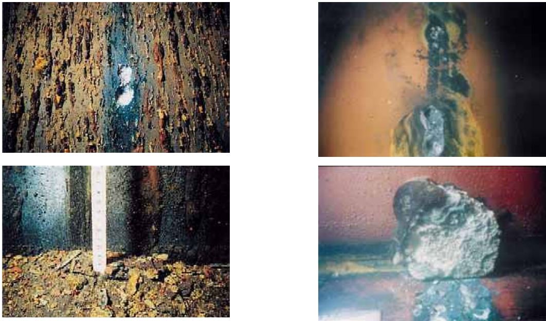
Figure 12 Various corrosion patterns seen in heat storage tanks (courtesy of /7/)
