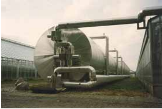
Figure 6 Horizontal heat storage at greenhouse cogen installation. The tanks used are in fact insulated tanks originally used for keeping heavy fuel oil at ready-to-use temperature.
