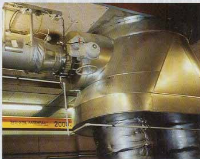
Pre-purge system for flushing the exhaust and dilute flue gases during start/stop sequence
