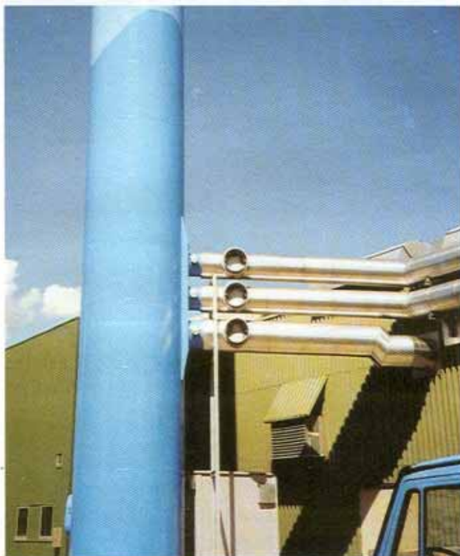
Vacuum valves at the chimney inlet to prevent collapse of the inner tubing during stoppage
