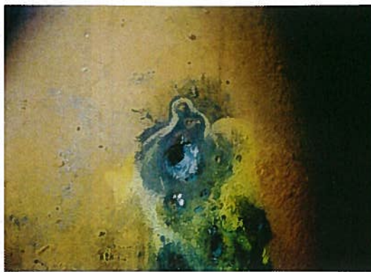
Corrosion patterns in heat storage tanks. PHOTO: J.H. Dyk
