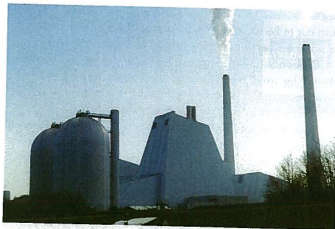
Heat storage tanks at a multi-fuel (coal, natural gas, oil, wood chips, straw) cogeneration unit
