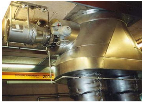
Figure A.2.1: Vent for flushing the exhaust system at start or stop
