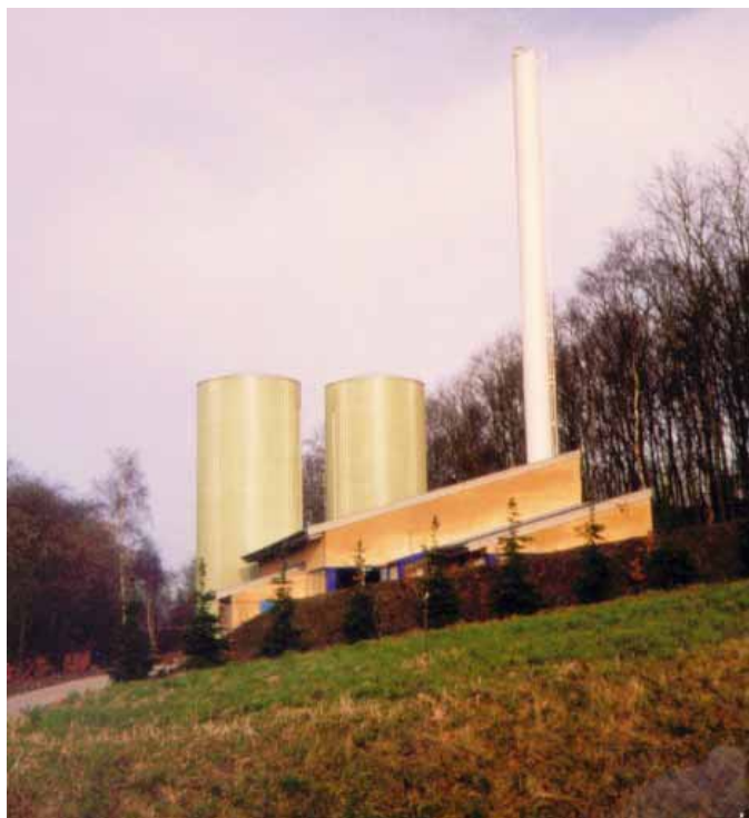
Figure 9 Two heat storage tanks installed next to each other at a hill-side gas-engine based cogen plant
