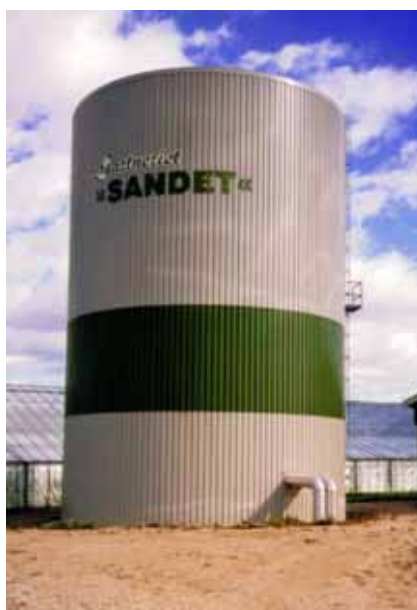
Figure 17 Heat storage tank at the greenhouse "Sandet" - as clearly shown
