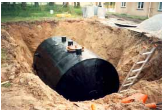
Figure 7 Underground horizontal heat storage tank for a small domestic cogen installation
